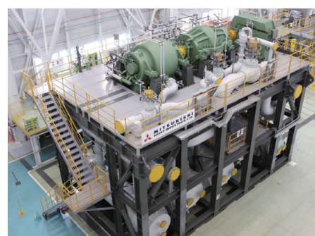
Nitrogen injection compressor module for ASU Plant
