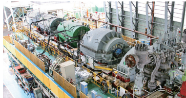
Cracked gas compressor train for mega ethylene plant
