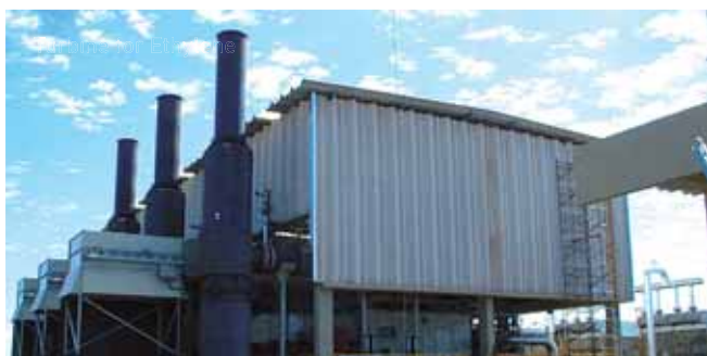
Gas Pipeline Station
