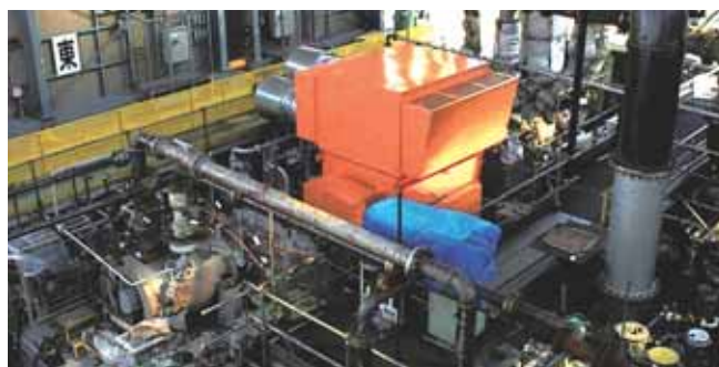
Carbon Dioxide re-Injection Compressor
