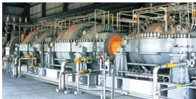
Cracked Gas Compressor & Steam Turbine for Ethylene
